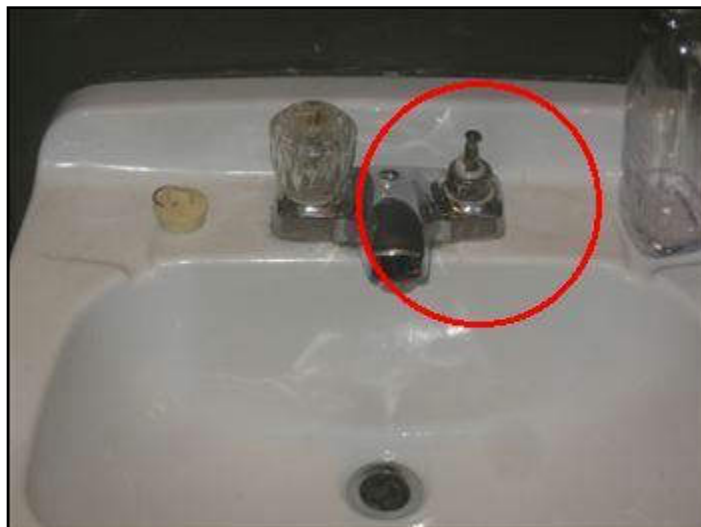
15. Missing faucet handle
