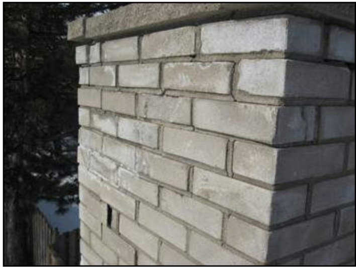
12. Loose and deteriorated masonry
