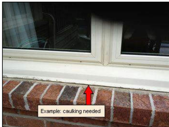
4. Caulking missing, loose or deteriorated
